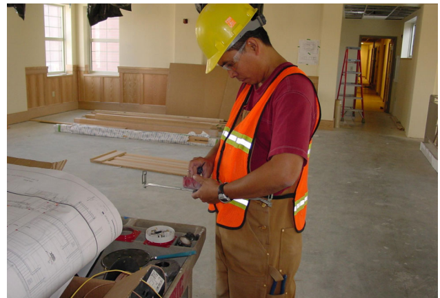
Ricardo Garces working on the Fire Alarm System at the Fort Lewis Barracks project.
